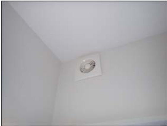
Lighting fixture and ventilation fan on wall. Operation was tested and working OK.
