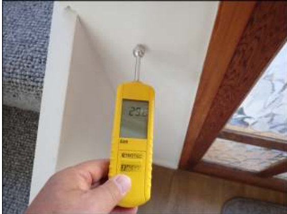
Photo 28.1 Normal level of moisture detected on wall facing exterior at foyer area. Optimal level shall be between 20 and 40.
