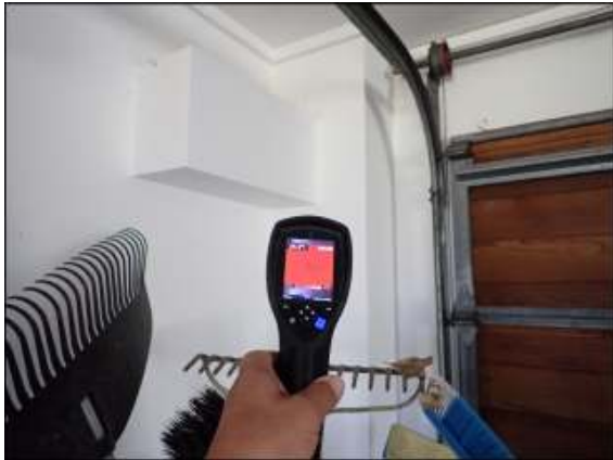
Photo 26.3 Normal level of moisture reading detected with infrared thermal imaging camera on wall facing exterior in garage.
