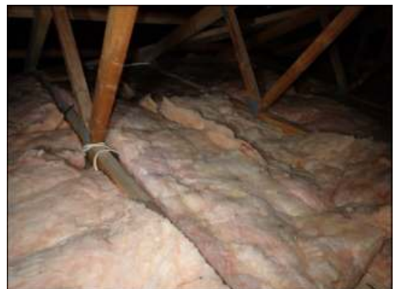
At attic(roof cavity), fibreglass blanket insulation laid in with R-1.8 approximately.
