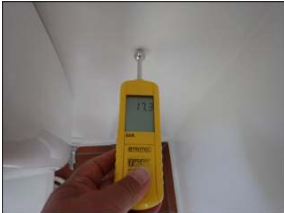
Normal level of moisture detected on wall around toilet. Optimal level shall be between 20 and 40.
