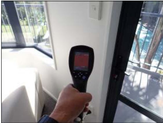
Photo 27.3 Normal level of moisture reading detected with infrared thermal imaging camera on wall facing exterior in family room.
