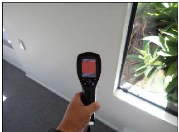
Photo 25.6 Normal level of moisture reading detected with infrared thermal imaging camera on wall facing exterior at kitchen/dining area.
