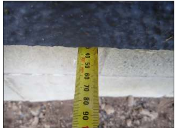
Bottom of of EIFS(Exterior Insulation & Finish System) exterior wall cladding appeared in good condition without damage or anomaly noticed.
