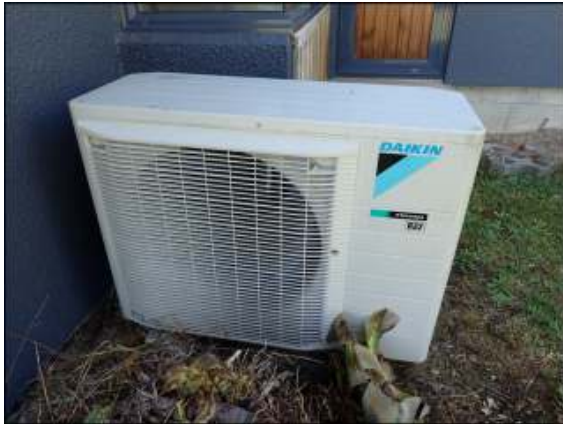
8.0 kW heating capacity heat pump generator on pad appeared in good condition. Operation was not tested.
