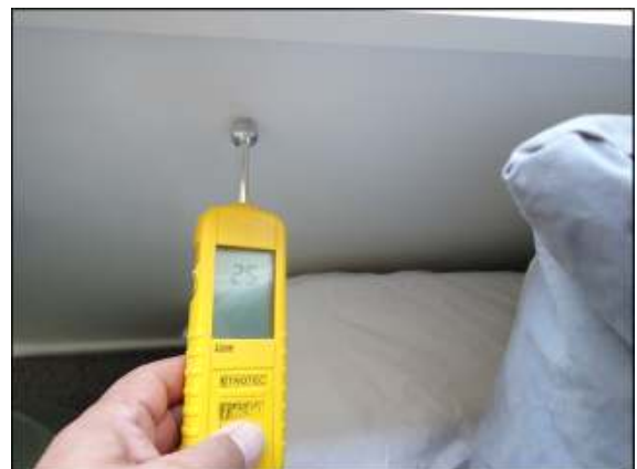
Photo 29.6 Normal level of moisture detected on wall facing exterior in bedroom III. Optimal level shall be between 20 and 40.
