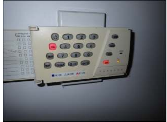
Home security control panel on interior wall. Operation was not tested.
