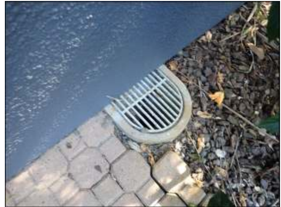
Raised with concrete gully trap secured with metal lid appeared in good condition.
