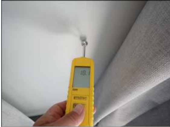
Photo 30.1 Normal level of moisture detected on wall facing exterior in bedroom IV. Optimal level shall be between 20 and 40.
