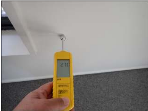
Photo 30.3 Normal level of moisture detected on wall facing exterior in family room. Optimal level shall be between 20 and 40.
