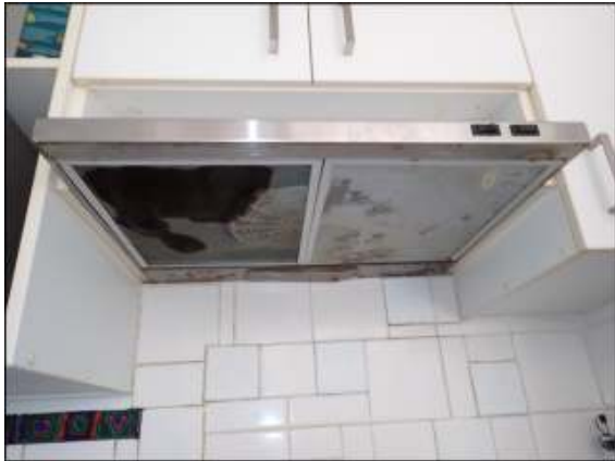
Ventilation fan and lighting fixture above cook top. Operation was not tested.
