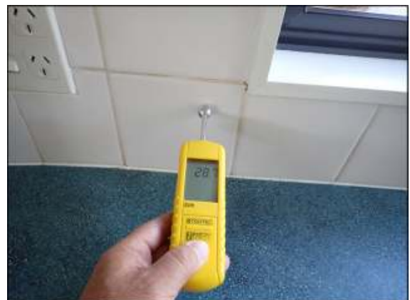
Photo 28.6 Normal level of moisture detected on wall facing exterior at kitchen/dining area. Optimal level shall be between 20 and 40.
