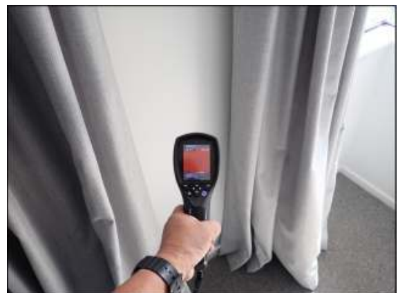
Photo 27.6 Normal level of moisture reading detected with infrared thermal imaging camera on wall facing exterior in master bedroom.
