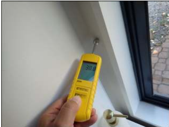
Photo 28.3 Normal level of moisture detected on wall facing exterior in bedroom II. Optimal level shall be between 20 and 40.
