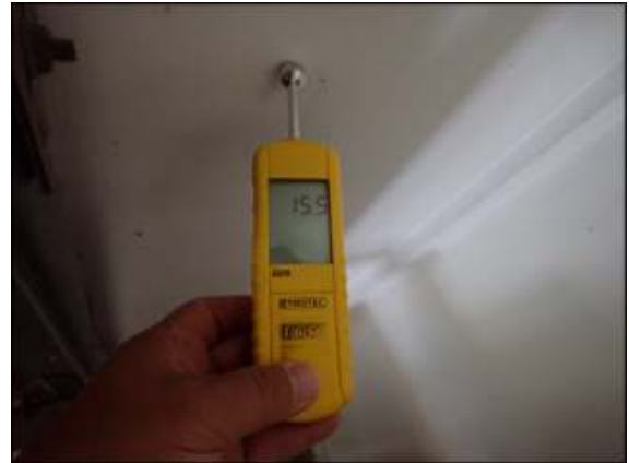
Photo 29.4 Normal level of moisture detected on wall facing exterior in garage. Optimal level shall be between 20 and 40.
