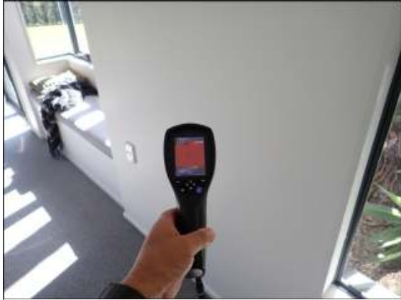
Photo 26.1 Normal level of moisture reading detected with infrared thermal imaging camera on wall facing exterior around living room.
