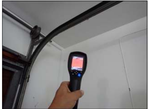
Photo 26.4 Normal level of moisture reading detected with infrared thermal imaging camera on wall facing exterior in garage.
