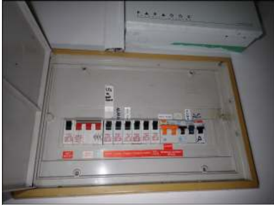
Electric power distributor and circuit breaker. No damage or risk factor noticed.
