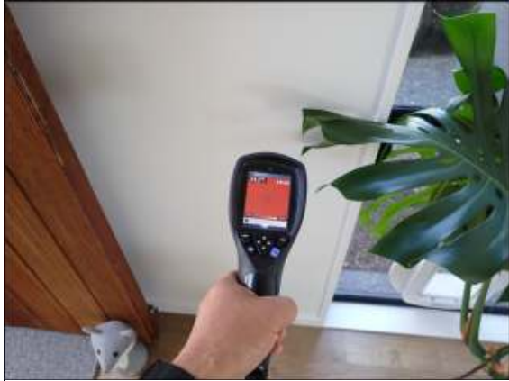
Photo 25.1 Normal level of moisture reading detected with infrared thermal imaging camera on wall facing exterior at foyer area.
