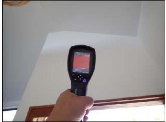
Photo 25.2 Normal level of moisture reading detected with infrared thermal imaging camera on wall facing exterior at foyer area.
