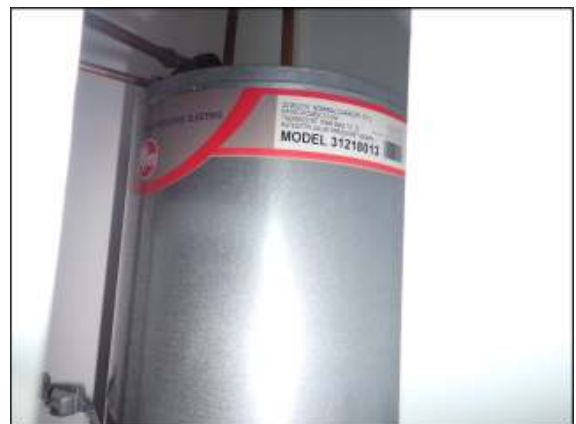
177 litre electric mains pressure hot water heater, manufactured in June 2016.
