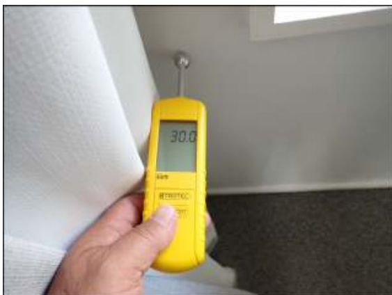
Photo 29.5 Normal level of moisture detected on wall facing exterior in bedroom III. Optimal level shall be between 20 and 40.
