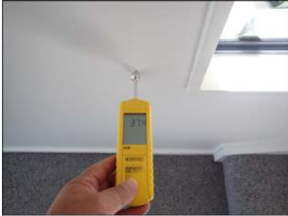
Photo 29.1 Normal level of moisture detected on wall facing exterior in living room. Optimal level shall be between 20 and 40.
